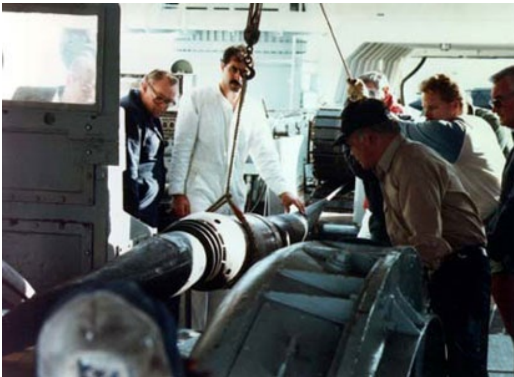
Photo of laying cable for TAT-8. Laying cable and a repeater for TAT-8 from the deck of the CS Long Lines, 1987.
