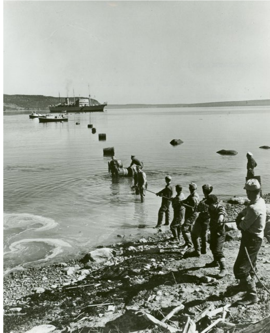
Transatlantic Cable (TAT-1) Under Construction, 1955. When AT&T opened TAT-1 in 1956, the first trans-Atlantic telephone cable, the initial capacity was 36 calls at a time.
